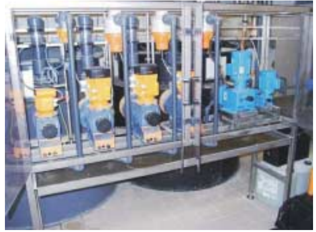
Dosing pumps for concentrate and disinfection.
